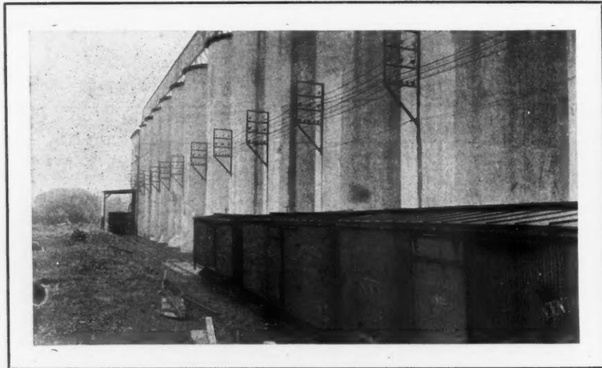
All the new Silos, numbering 45 in all—a new Packhouse and a new Baghouse have been built by Burrell for the Lawrence Portland Cement Co. at Siegfried, Pa. Four more Silos now under construction.
